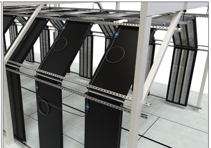
LEINS3 shown with DALI cabling
